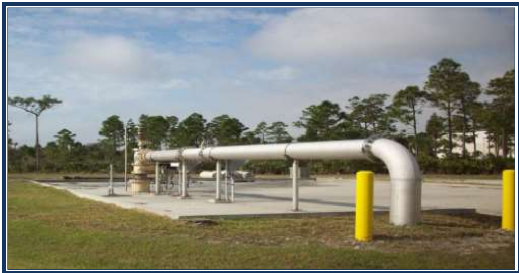
Injection Well #2 Tropical Farms
