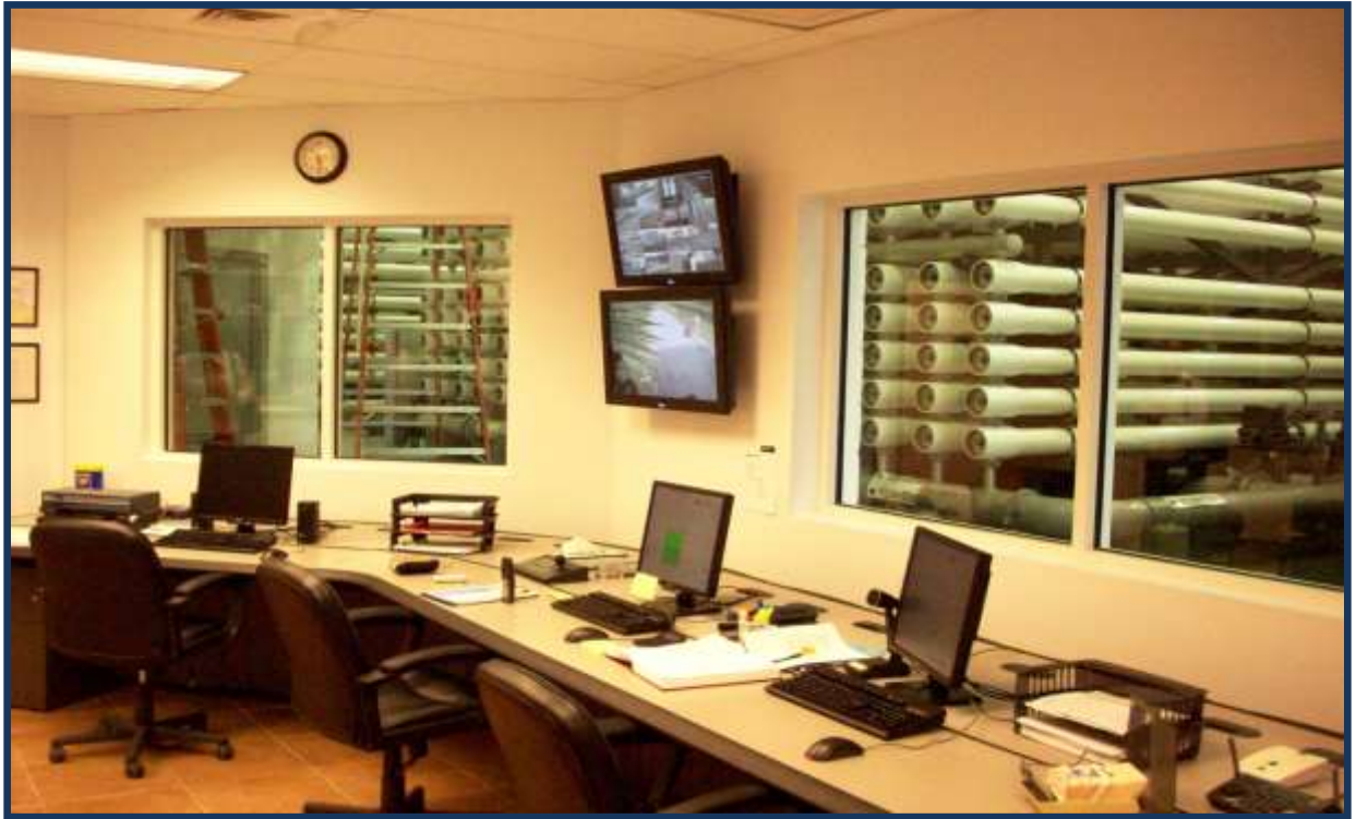
Control Room Tropical Farms Operations Building
