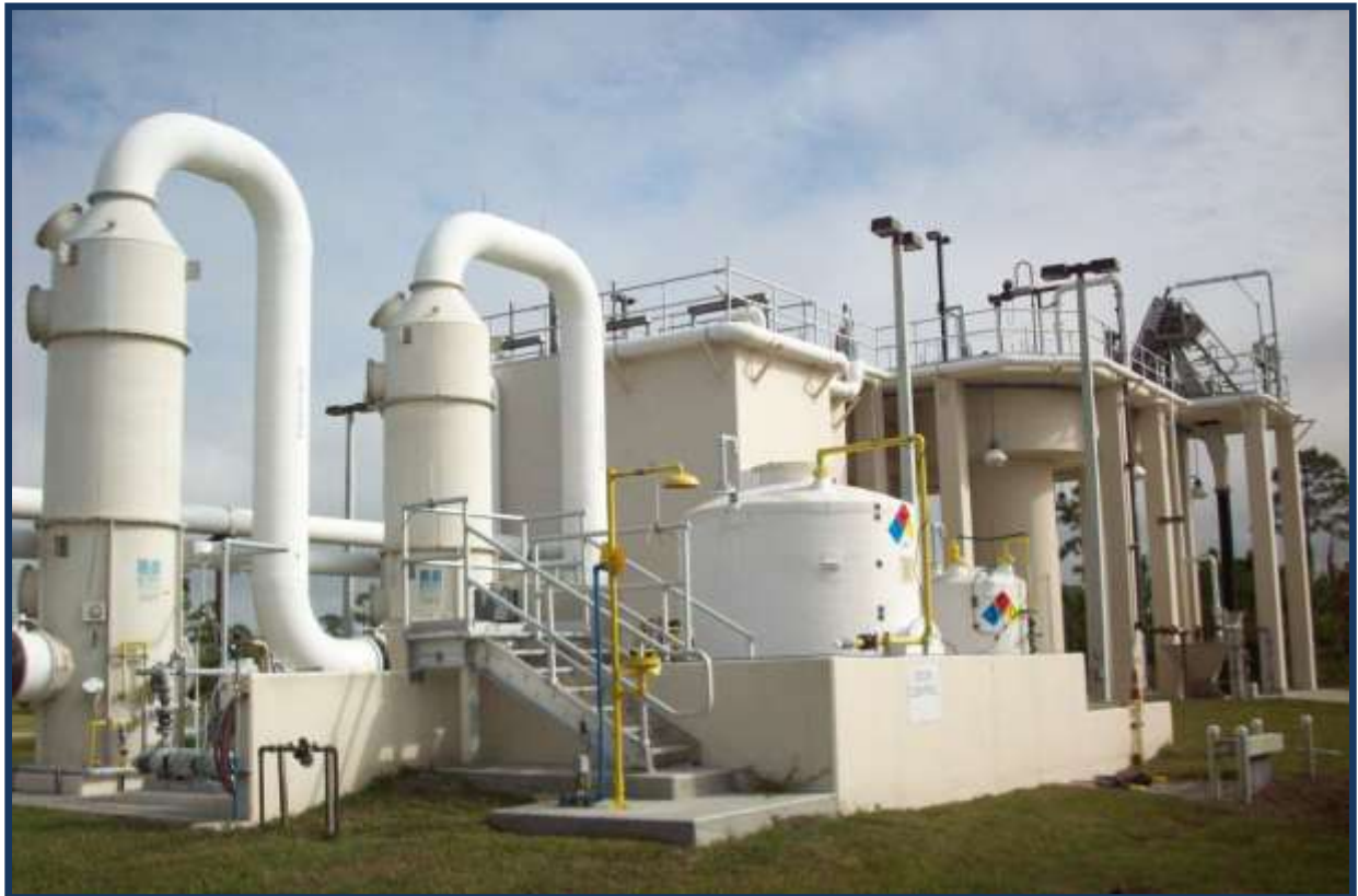
Head Works and Odor Control Tropical Farms Wastewater Plant
